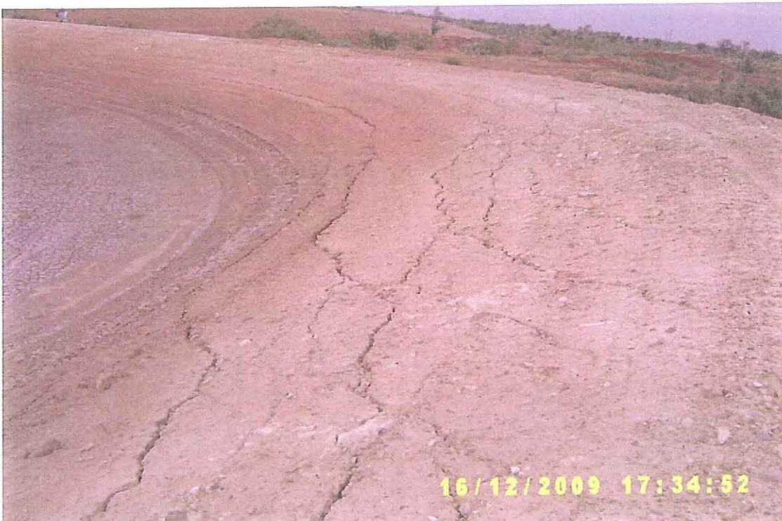
Photo 4: Cracks within Evaporation/Water Dam Embankments.
