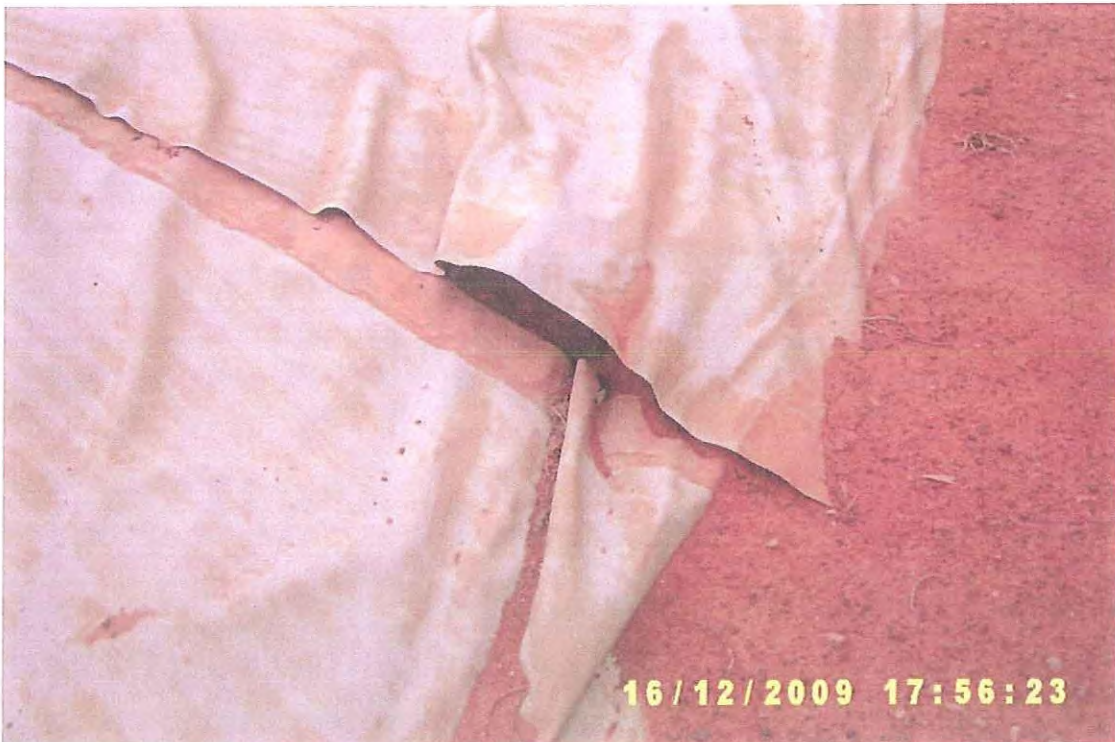
Photo 6: Perished Seams of the Bulk Fuel Storage Facility Liner
