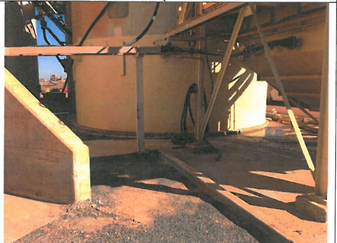
Photograph 4 – Water leak from an old unused leachate tank
