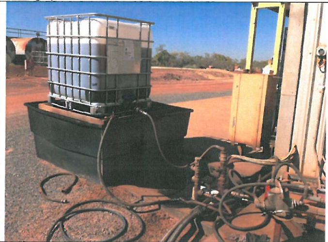
Photograph 21 – Small exhaust spill at power generation station
