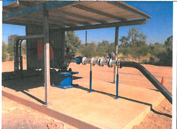
Photograph 16 – Pit 2 pump station
