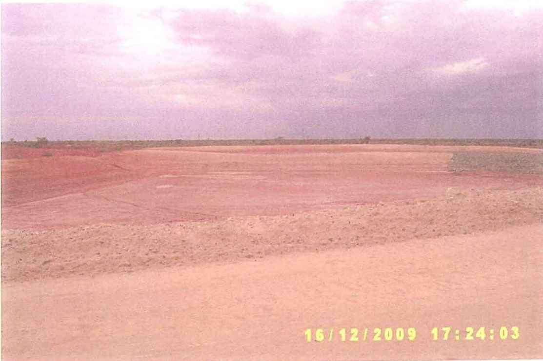
Photo 3: Evaporation/Water Dam constructed without approval.
