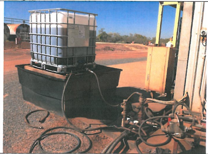
Photograph 21 – Small exhaust spill at power generation station
