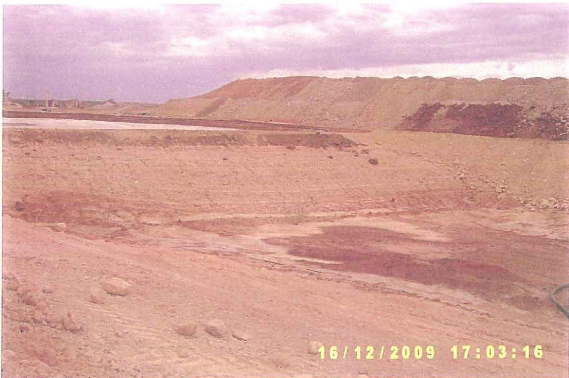
Photo 2: Seepage Visible on External Embankment Wall of TSF 2.
