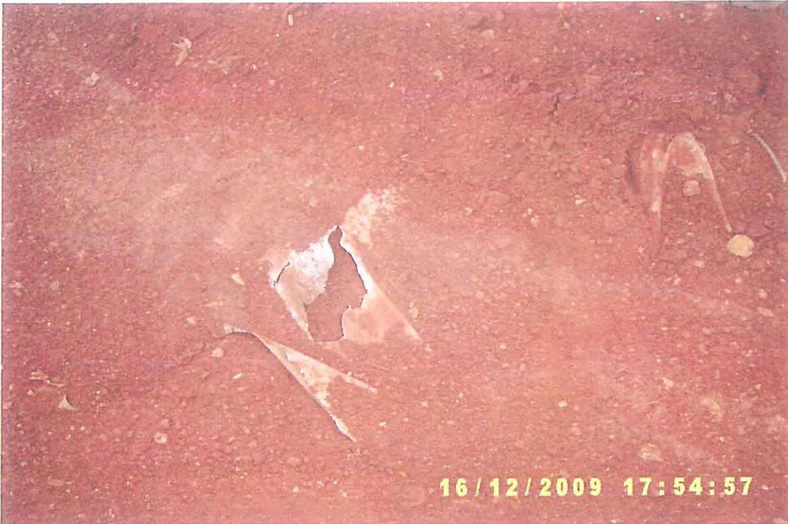
Photo 5: Tears within the Bulk Fuel Storage Facility Liner
