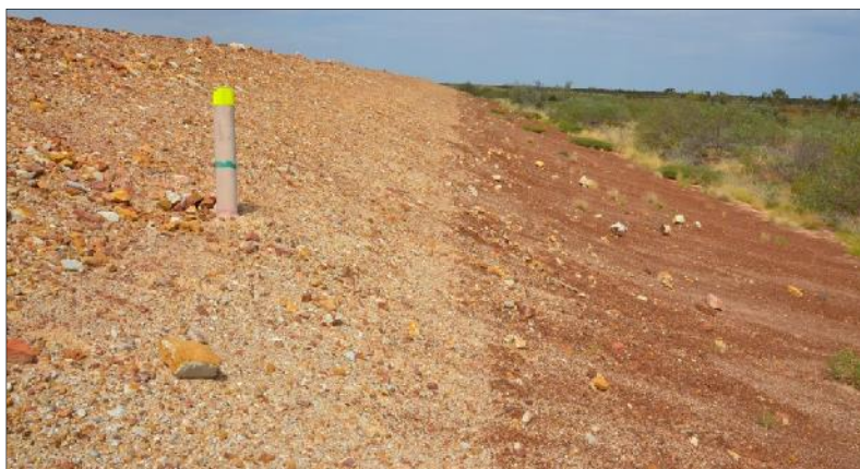
Plate 10: Vibrating wire piezometer PT2N, Cell 2 northern downstream embankment face
