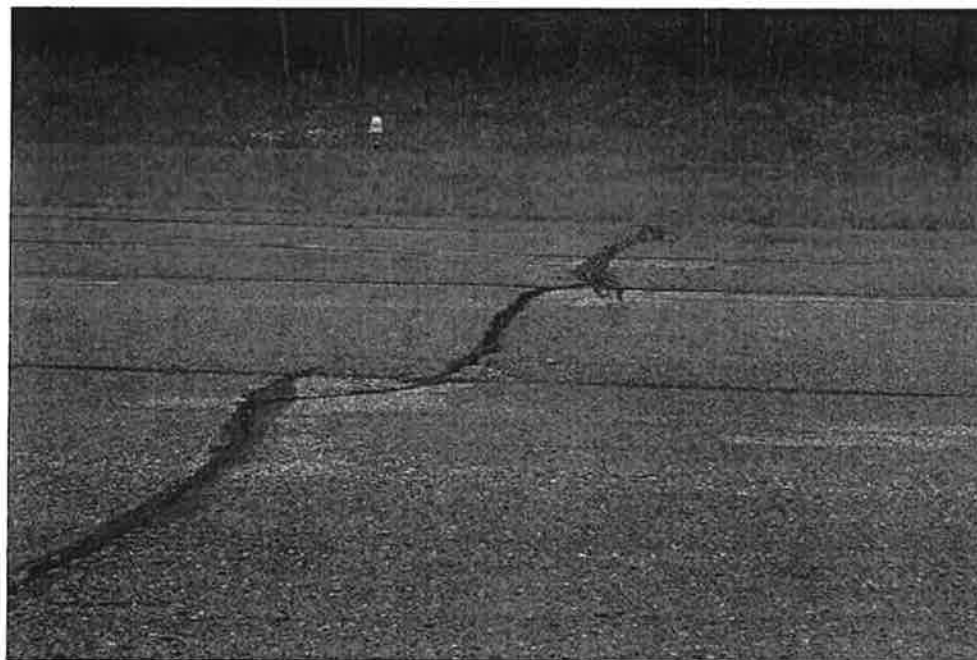
Photograph 4: Typical transverse crack on Runway 09-27.
