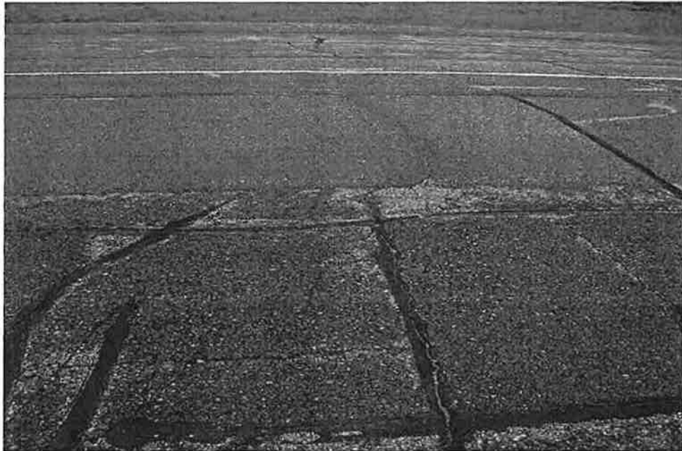
Photograph 5: Typical crack pattern on Runway 09-27.
