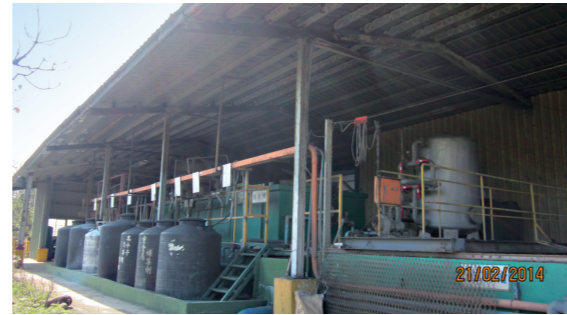
▲ Taoyuan 1st Plant waste treatment Plant
