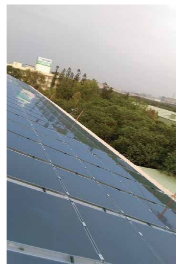
Solar PV system installed in Taoyuan 1st Plant
