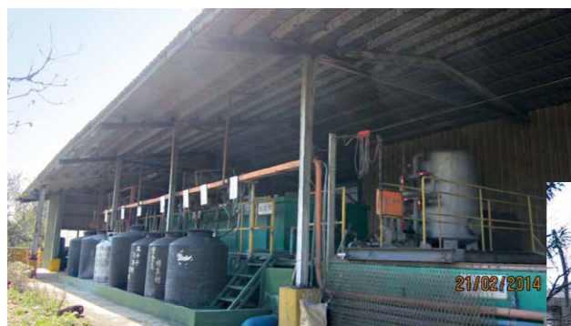
Taoyuan 1st Plant waste water treatment Plant
