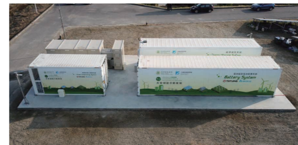
▲ Power storage system in Yong-An, Kaohsiung City
