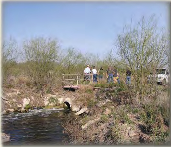
Wastewater outfall, Mission
