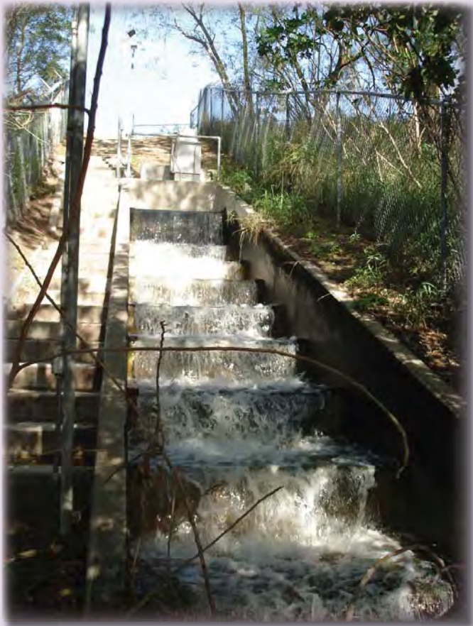
Wastewater outfall in Harlingen
