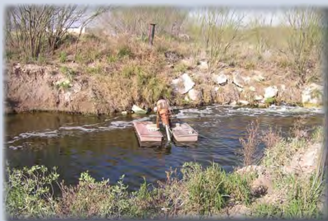
Floating aerator, Mission wastewater outfall
