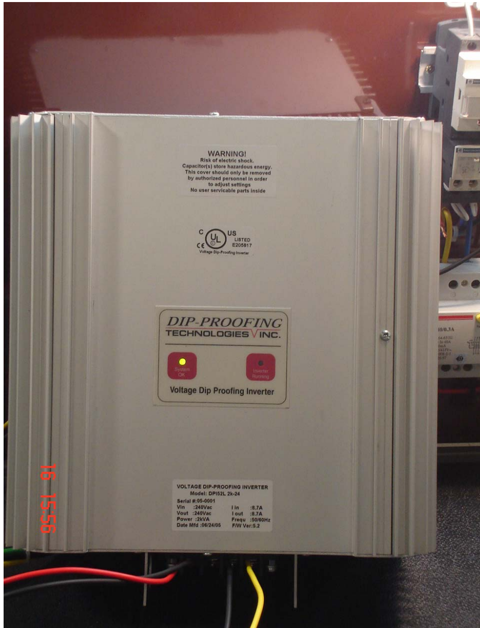
Figure 32: Dip Proofing Inverters (DPI)
