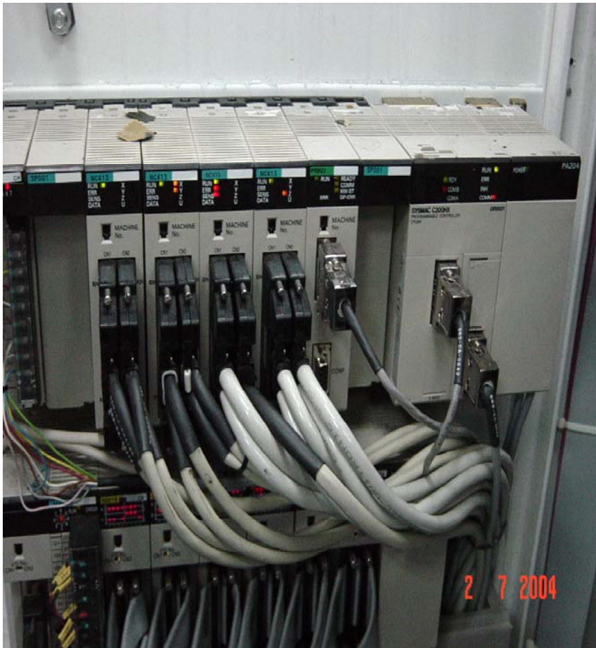
Figure 15: Programmable Logic Control (PLC)
