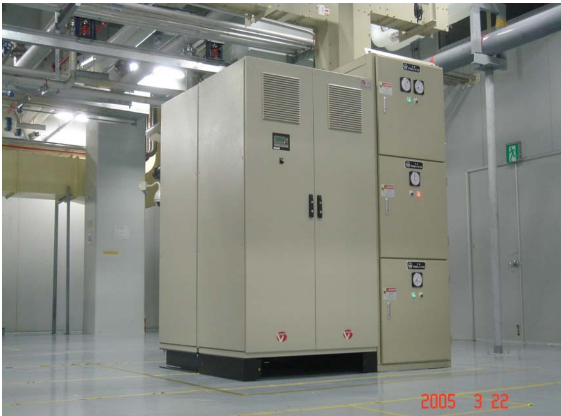
Figure 36: Active Voltage Conditioner
