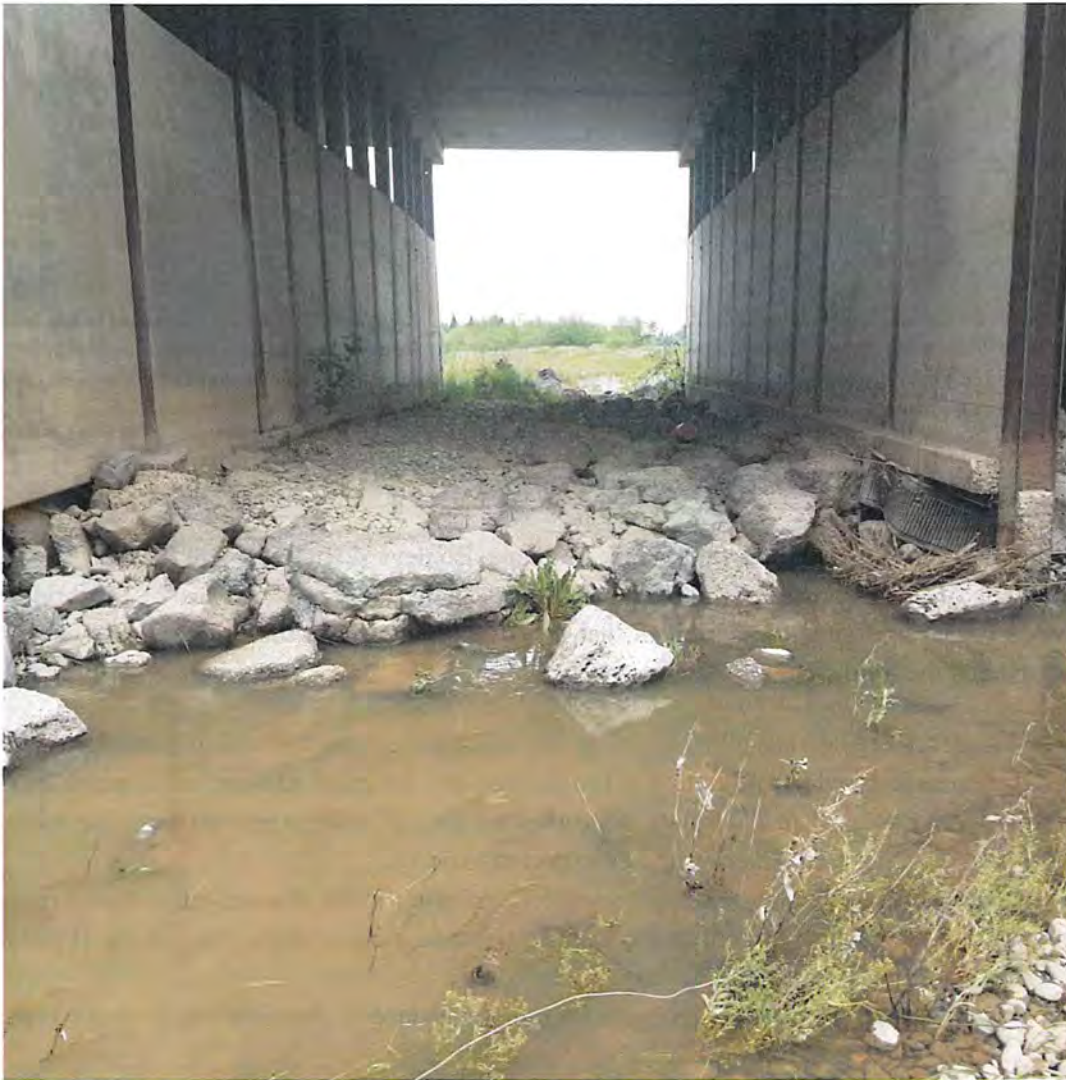
Photo 2-7: Existing concrete and rock between two bridge bents under the Antelope Boulevard/Highway 36 Bridge.
