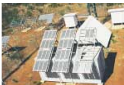
← Telstra's repeater stations, such as this one at Six Mile Creek in NT, are fundamental to Telstra's network serving rural Australians.
