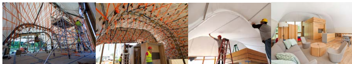
Figure 1: Four Stages of Construction: Ratchet Straps, Vapor Barrier, Light-Block Textile, and Interior Finish Textile
