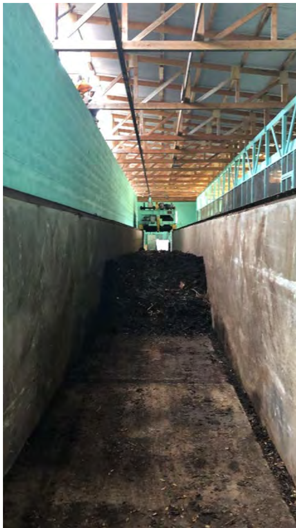
Figure 12: Composting chamber at the National Redemption Center, Palau. (Source: APWC, 2019)
