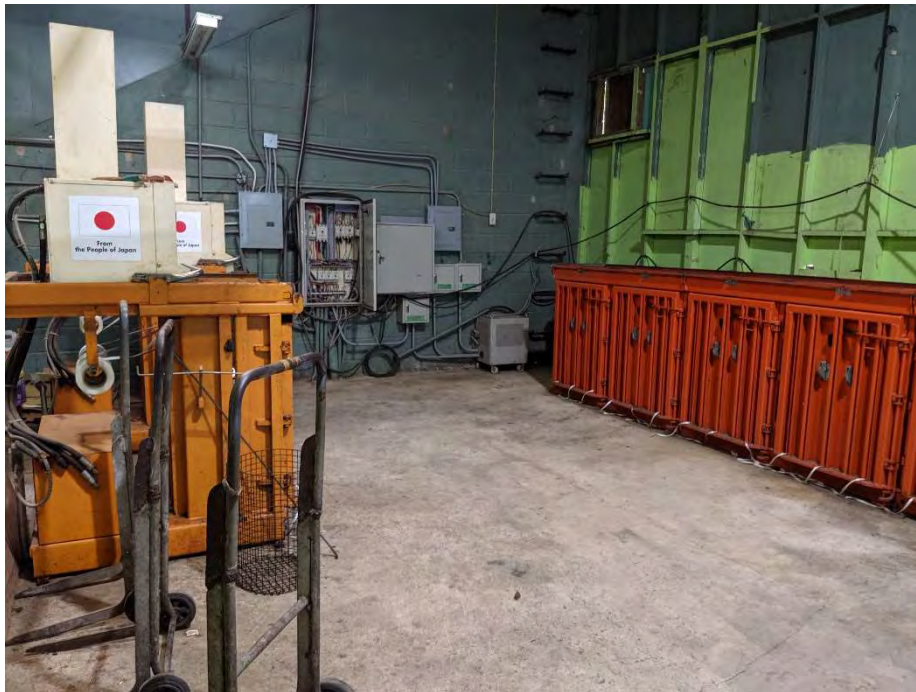
Figure 7: Baling machine at the National Redemption Center, Palau. (Source: APWC, 2019)
