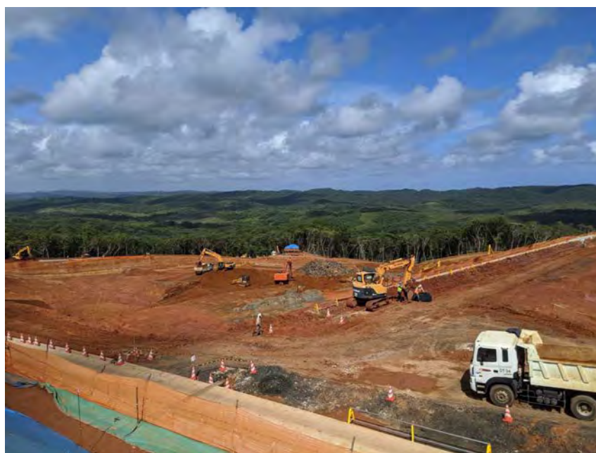
Figure 16: Construction underway at the national landfill in Aimeliik State. (UNEP Consultant team, November 2019)
