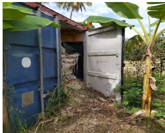
Photo 10. DDT stockpile container #2 vandalised
