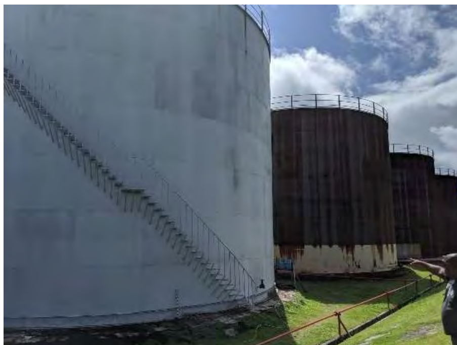
Figure 52: Palau Public Utilities Cooperation waste oil stockpile tanks. (Source APWC)
