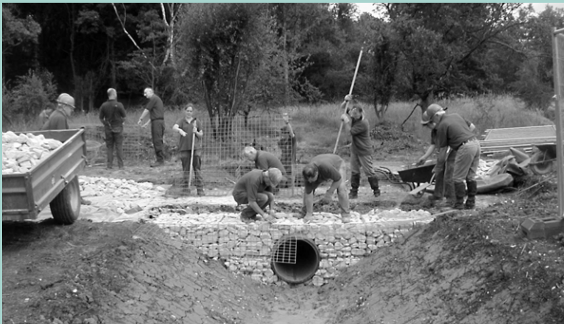
Volunteers constructing the flood control structure which will be soon be hidden by vegetation
