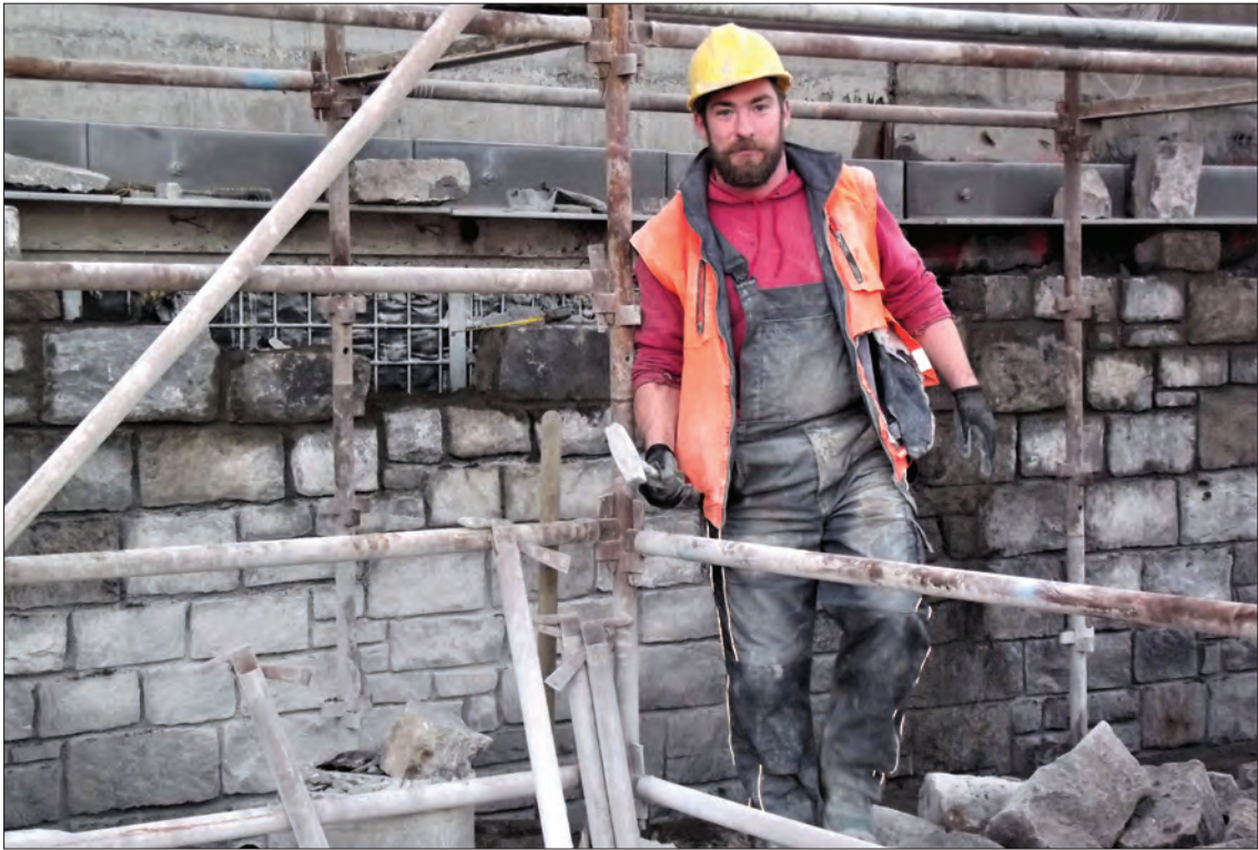
Illus. 4.2—Jason Ronayne, stonemason, at work on the new Clydagh Bridge in spring 2016.
