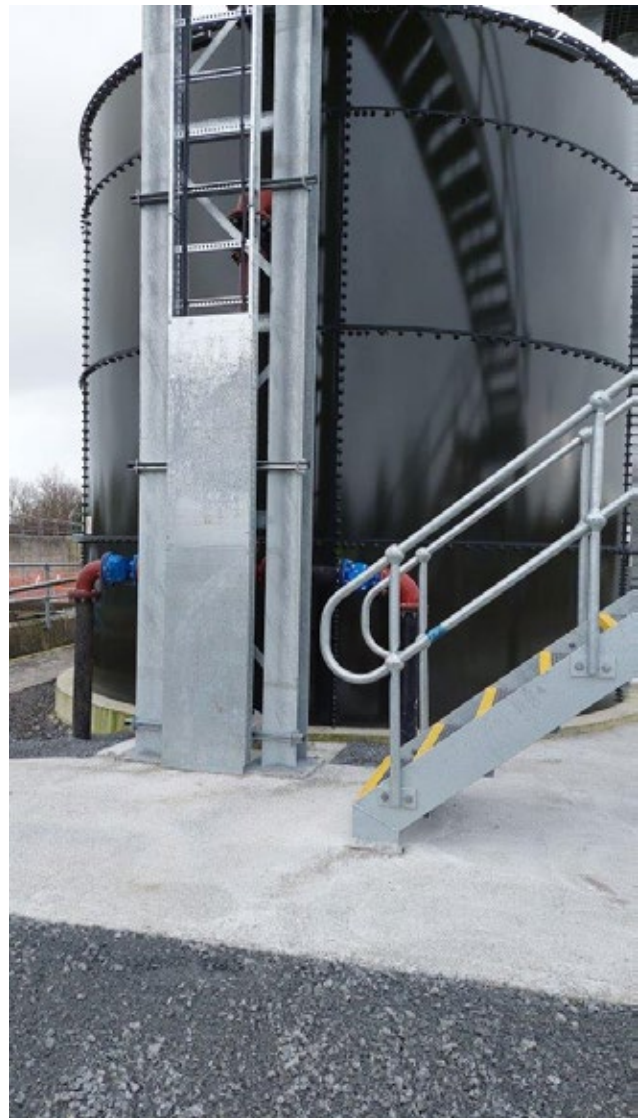
Borrisokane Wastewater Treatment Plant Upgrade
