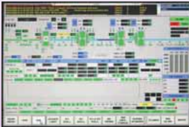
Operator's HMI Screen
