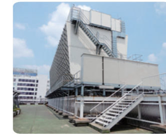
Nishi-Ikebukuro Heat Supply Facility
