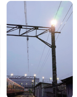
Minamikurihashi Vehicle Precinct Lighting fixtures in Kasukabe Branch Office
