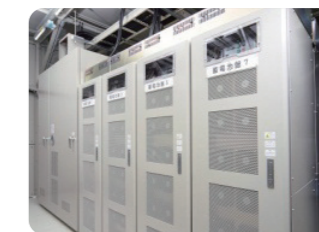
Regenerative power storage device
