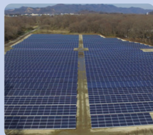
Tobu Iwafune Solar Power Plant (Tobu Energy Management)
