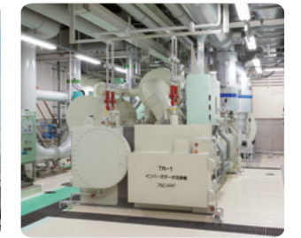
Kinshicho Heat Supply Facility
