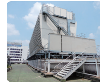
Nishi-Ikebukuro Heat Supply Facility
