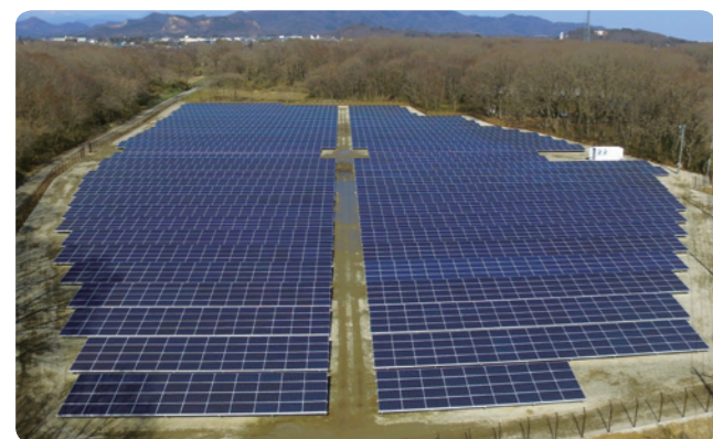
Tobu Iwafune Solar Power Plant
