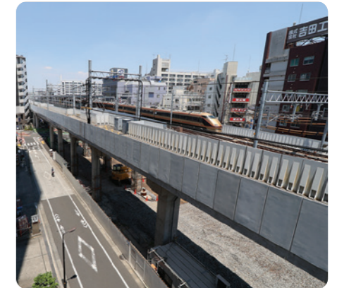
FRP sound insulation wall (bridge railing)
