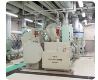
Kinshicho Heat Supply Facility
