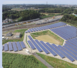
Tobu Takayanagi Solar Power Plant (Tobu Energy Management)
