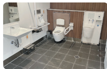
Barrier-free restroom (Shinkiryu Station)
