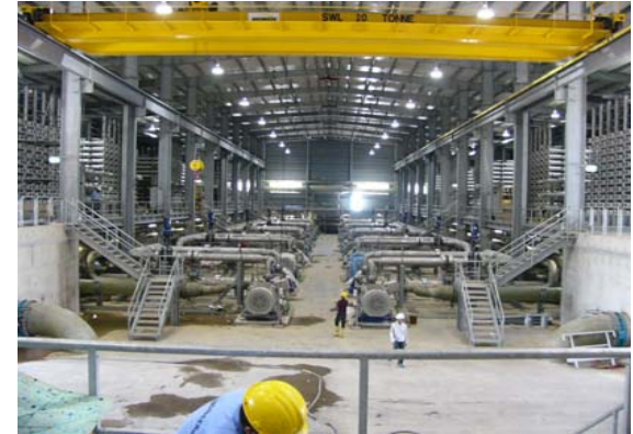
The SingSpring Desalination Plant in Singapore built by Hydrochem
