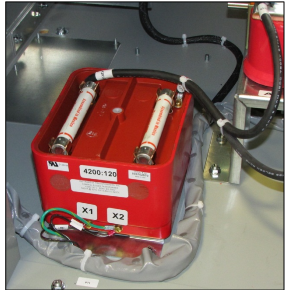
Fig. 27 Control Power Transformer
