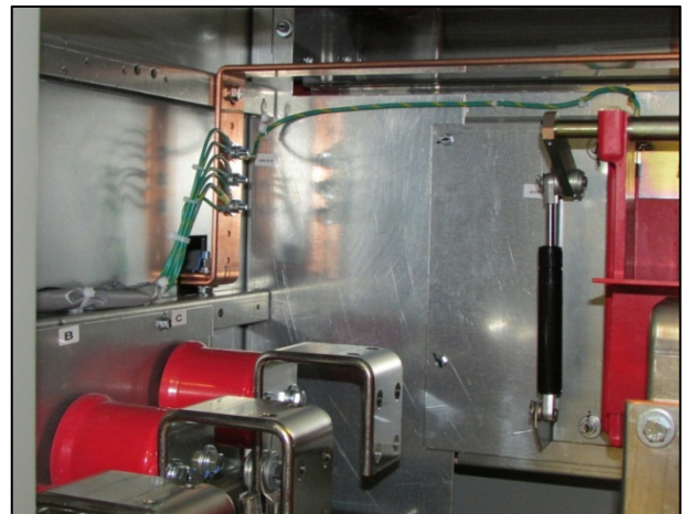
Fig. 8 Main Ground Bus
