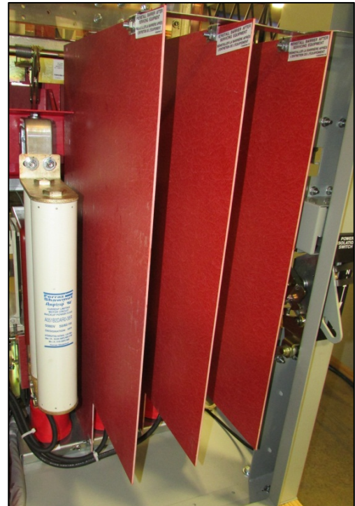
Fig. 45 Fuse Barrier Placement
