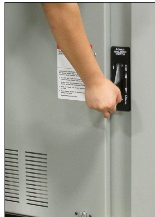
Fig. 39 Closing Isolation Switch
