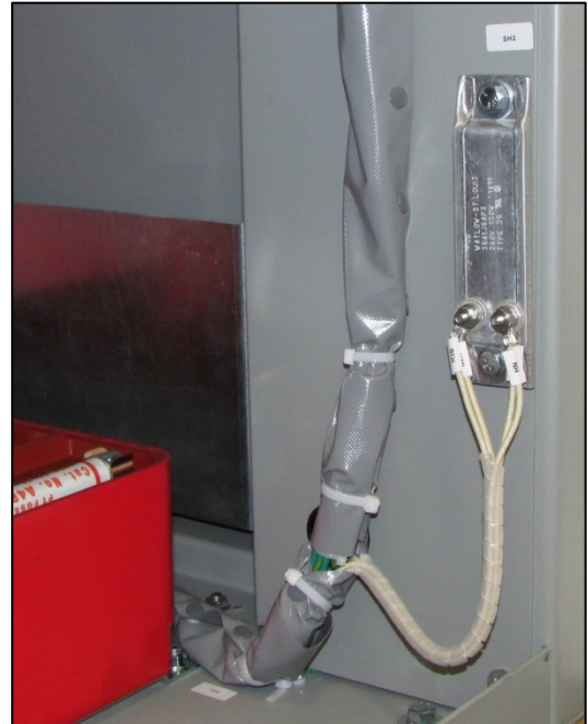
Fig. 5 Typical Space Heater
