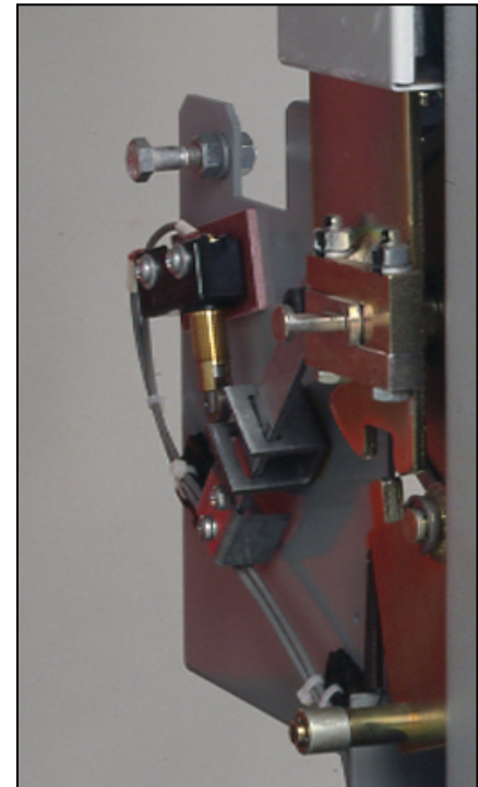
Fig. 9 Control Power Interlock
