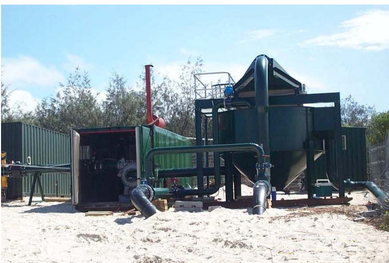
temporary onshore pump and slurry systems for transfer of extracted sand to the foreshore requiring renourishment.
