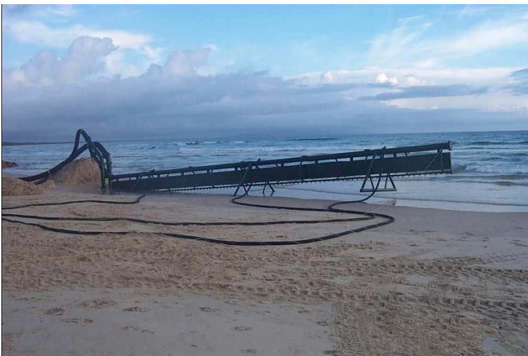
sand shifter unit: in the process of self submerging at the selected sourcing site
