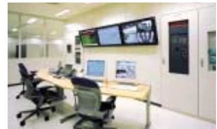
The machine room oversees the network connecting Toyota Industries' bases all over the world
