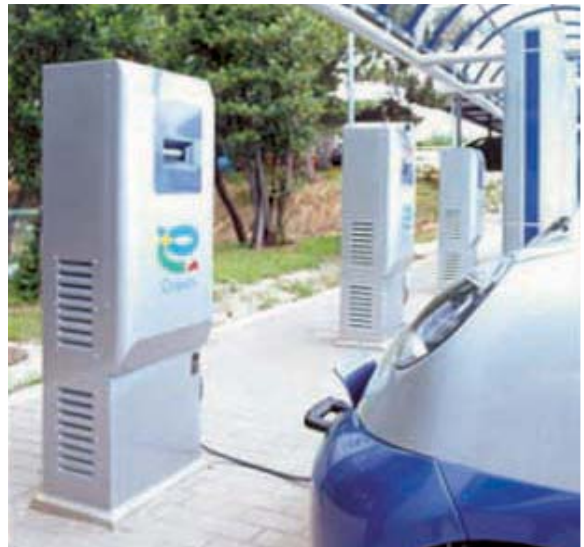
Battery Charging System for EV
