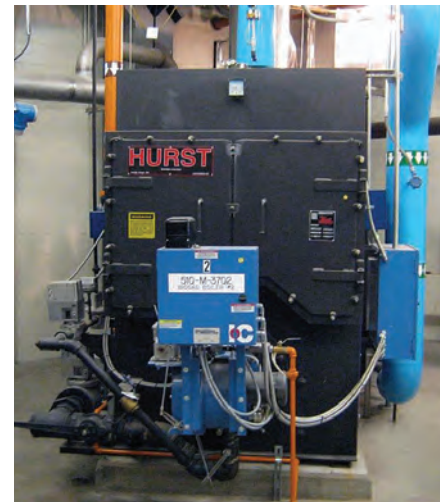
A pair of Hurst 5,000 MBH boilers will use biogas from the digesters to heat sludge before it enters the digesters to improve treatment efficiency.
