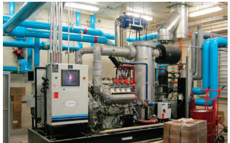
Two 275 kW cogenerator units will increase electrical generation at the plant and save about $300,000 a year (Gen-Tech). Recovering waste heat from the engines will also contribute about 20 percent of the plant’s heating needs.
