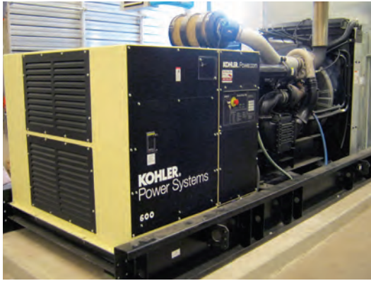
The Eau Claire facility also has two diesel-powered 600 kW emergency generators in the event of a power loss to the plant (Kohler).
