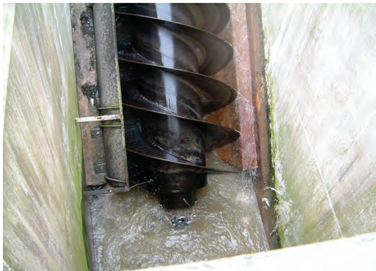
Figure 3. A modern labyrinth bearing protection seal on an Archimedean screw fitted in a wastewater treatment plant.
