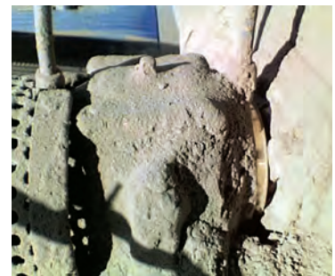
Figure 1. Labyrinth bearing seal (LabTecta 660AP) on a powder application. Air purge keeps the dust away from the stator to rotor interface.
