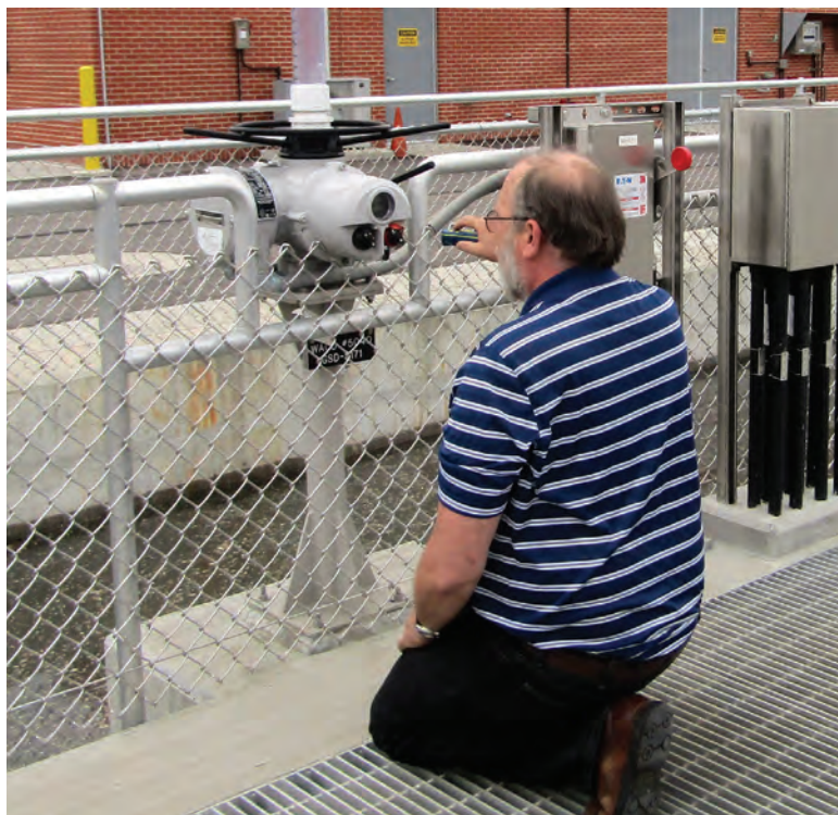
Acting superintendent Bill Young adjusts the wet weather clarifier's influent valve at the Springfield plant.
