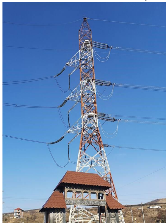
Photo: The 400/110/10 kV transformer substation Cluj Est
