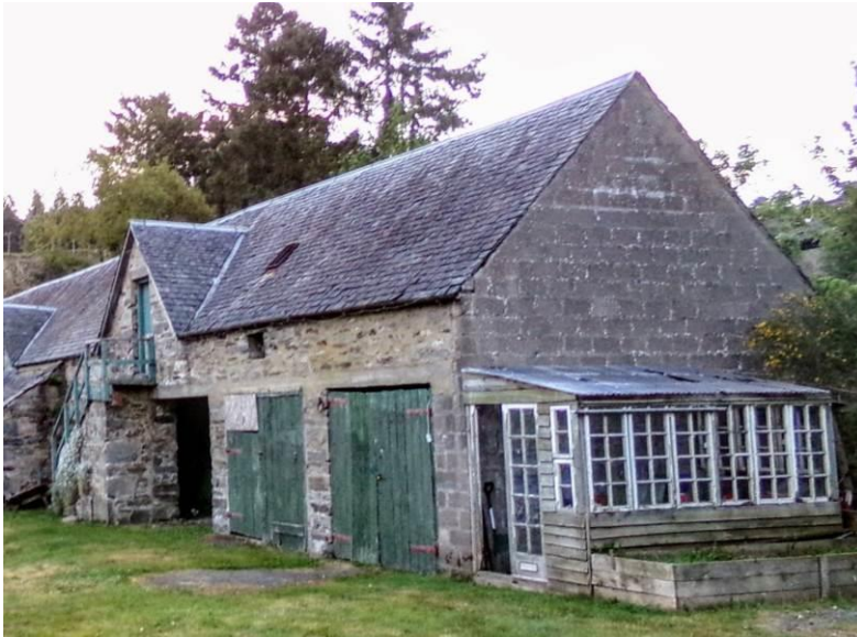
Photograph 13: Modern concrete block-work and lean-to, southern gable end of Guay Farmhouse Wing
