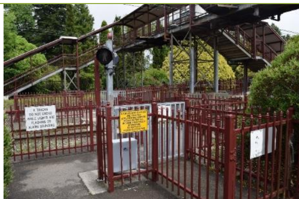
Figure 71 View of the level crossing and safety equipment
