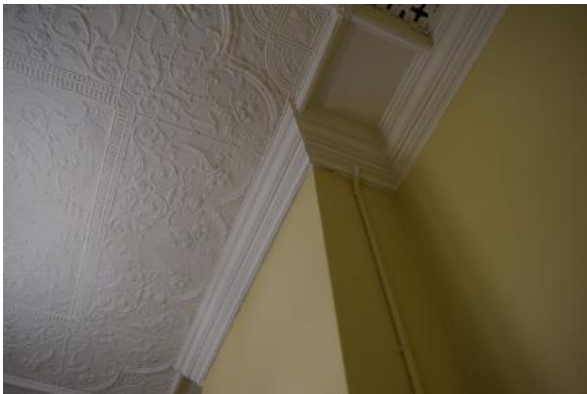
Figure 44 Closeup view of the north wall and ceiling junction and pressed metal ceiling
