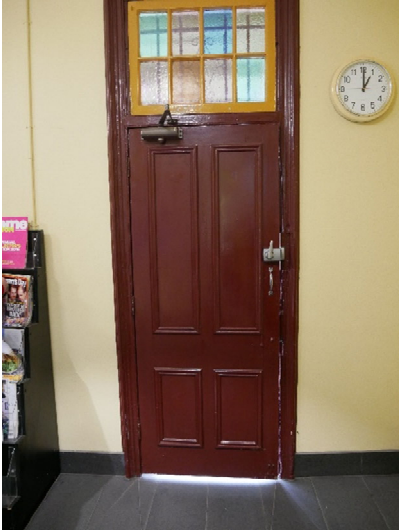
Figure 3536: Door D-01. (Source: Purcell, 15 October 2021.)
