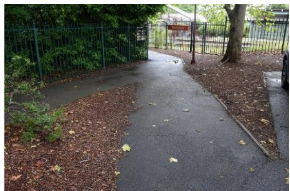
Figure 102 View of the footpath at the north extent of the car park leading to the footbridge
