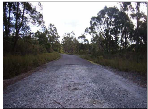
Segment L where it meets the existing sealed section that continues down to the Tayatea Bridge.
