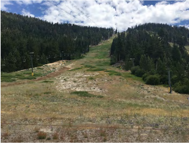
Before: Work in progress on covering gully with mulch on steep ski slope.
