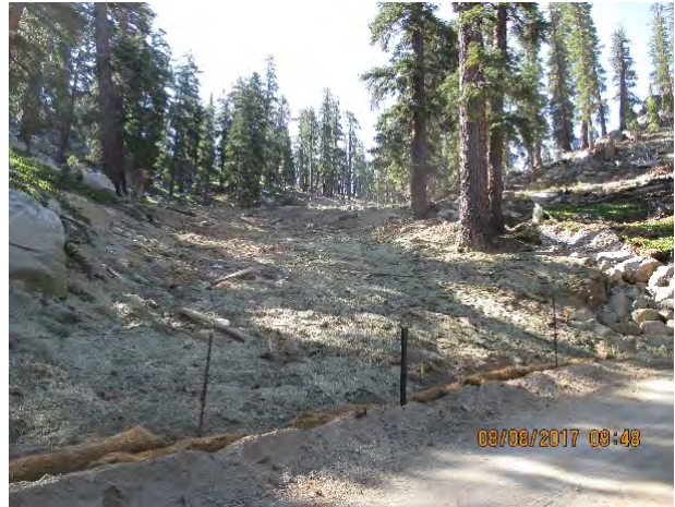
Hand Grenade Chute 2017 After: erosion resistance significantly improved on steep slope and toe of slope protection provided by cutoff ditch and pine needle wattle
