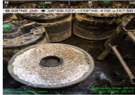
Loose clean media
