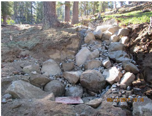
Hand Grenade Chute After 2017: rock riprap protection on gully with geotextile and covered culvert inlet to pass flows across roadway
