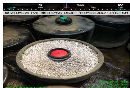
Loose clean media
