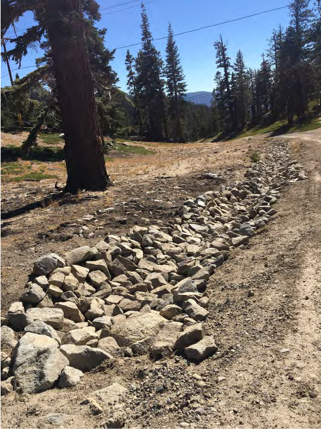
Trail Crew restored the Upper Shop Road rock line ditch – photo taken 9-25-18:
