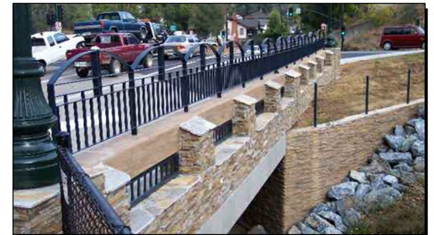
TYPE 80 BARRIER EXAMPLE WITH TIMBER TEXTURE AND STAIN ON TOP BEAM AND STONE VENEER ON POSTS AND BRIDGE DECK
