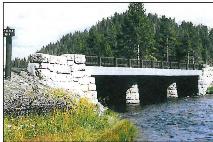
EXAMPLE OF DECORATIVE DARK BROWN RAILING AND LARGE BLOCK RUNNING BOND FORM LINER PATTERN ON COLUMNS AND WINGWALLS
