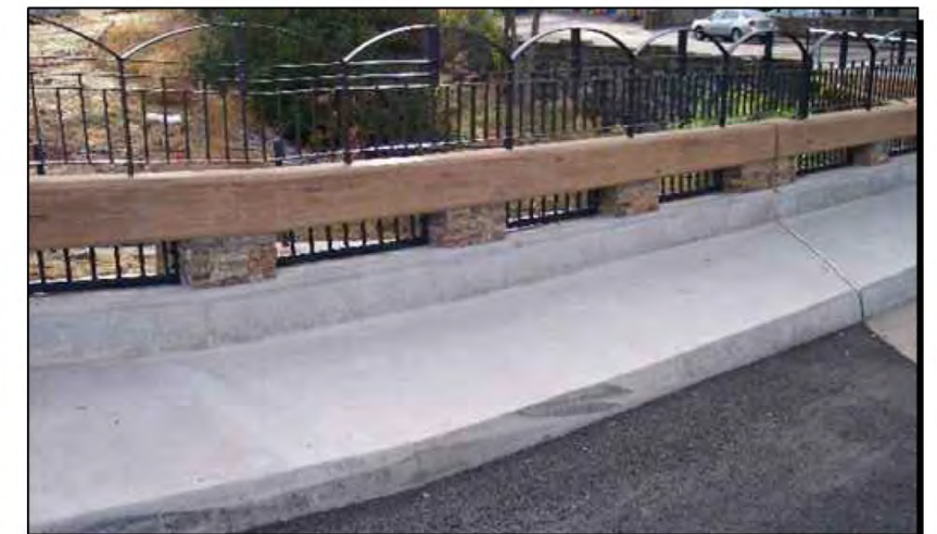
TYPE 80 BARRIER EXAMPLE WITH TIMBER TEXTURE AND STAIN ON TOP BEAM, STONE VENEER ON POSTS AND METAL PICKETS BETWEEN POSTS
