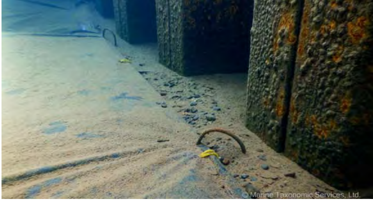
Benthic barrier installed with rebar staples at Fleur du Lac Outer Harbor
