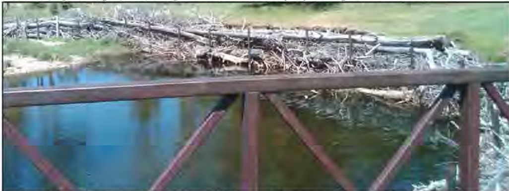
An undersized bridge on Hole 6 – the par 3. The logs placed horizontally are band-aids aimed at stopping the severe cut-bank erosion just downstream from the bridge. Just upstream from the bridge has been incised by the narrowing of the river.
