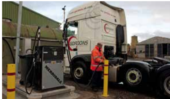
A road transport company's Merridale diesel fuelling point, with its ATEX-certified fuel pump on a separate island
