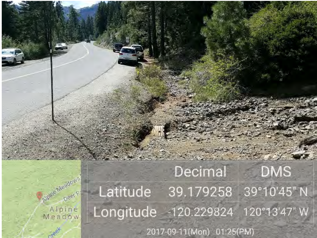
Figure 4-12 Sediment plugged culvert inlet, Alpine Meadows Road at Five Lakes Trailhead, Placer County, California.
