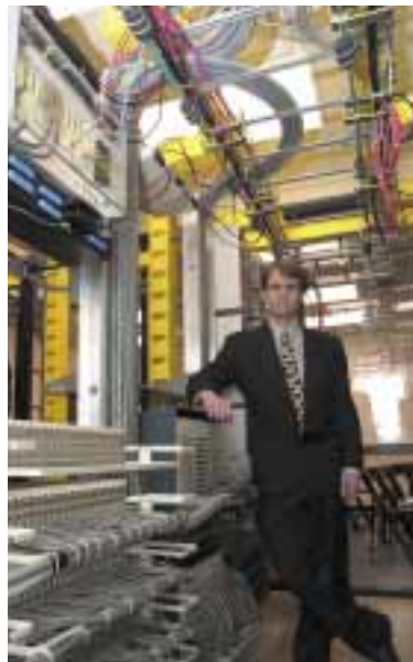
Electrical Engineering Professor Peter LoPresti stands in TU's new Williams Communications Fiber Optic Networking Laboratory, which opened in January. The lab, under LoPresti's direction, will be used by students learning how to design telecommunications networks, professional engineers seeking training on the latest equipment, and companies researching innovations that might further revolutionize the world of communication.
