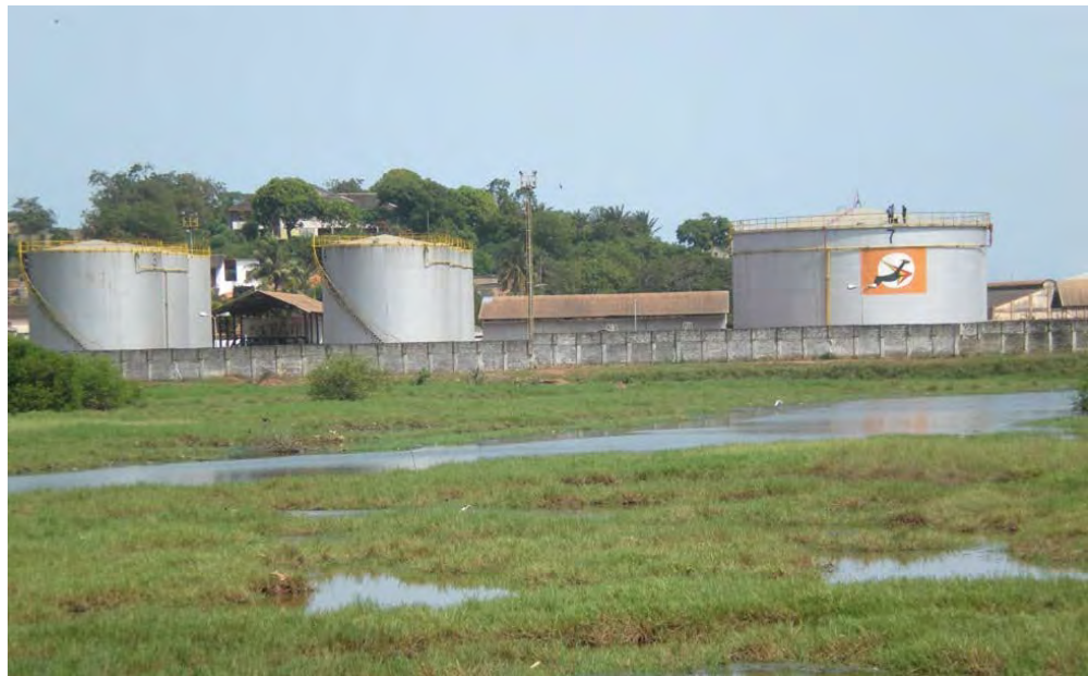
Figure 6.14 GOIL Bulk Fuel Storage in Takoradi
