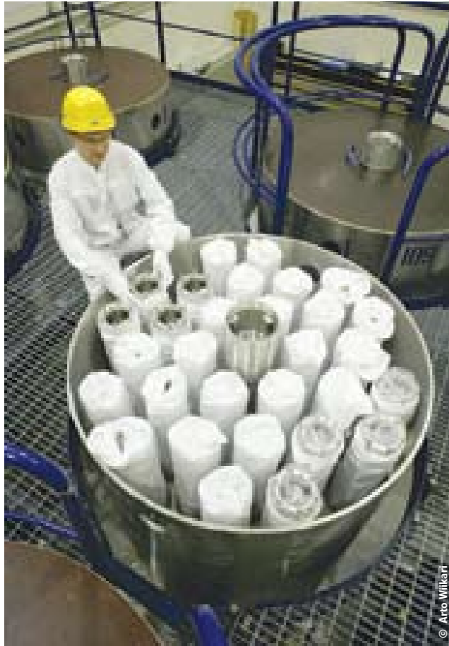
Figure 14-9. Fresh fuel assemblies in a transfer basket in the dry store of the Loviisa Power Plant.
