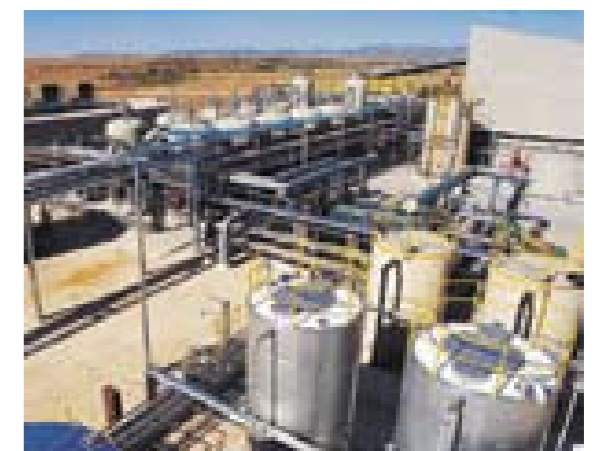
Figure 14-5. Beverley ISL production plant in Australia (Beverley).
