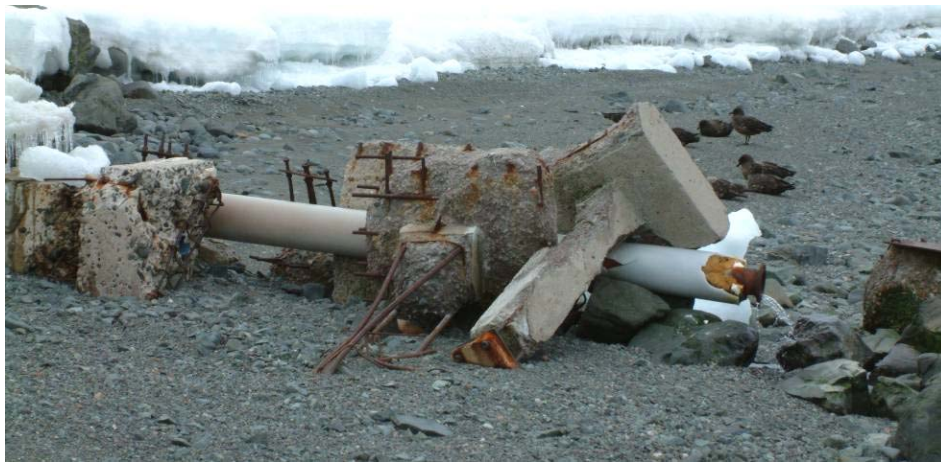
Fig. 4.3.-3: Exposed by low tide, Great Wall's waste water discharge pipe (photo: December 2003, Buesser)
