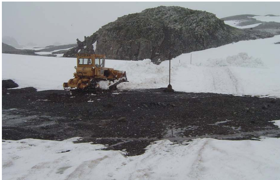
Fig. 4.2.-38: Important sections of the road network are cleared of snow if necessary. The way marking is then of particular importance (photo: Mustafa)
