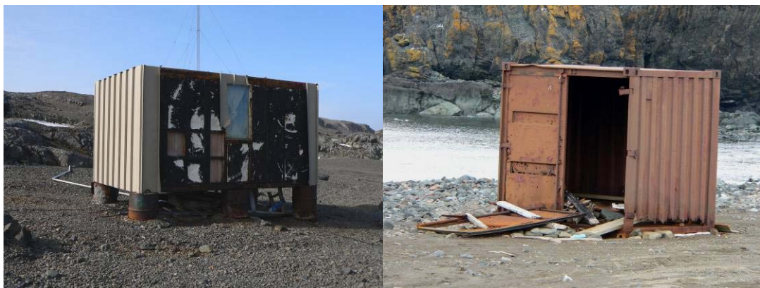
Fig. 4.2.-34a & b: Severely damaged containers on the east coast of the Fildes Peninsula (a) container near the Ardley Isthmus (b) container south of Great Wall (photos: Buesser)
