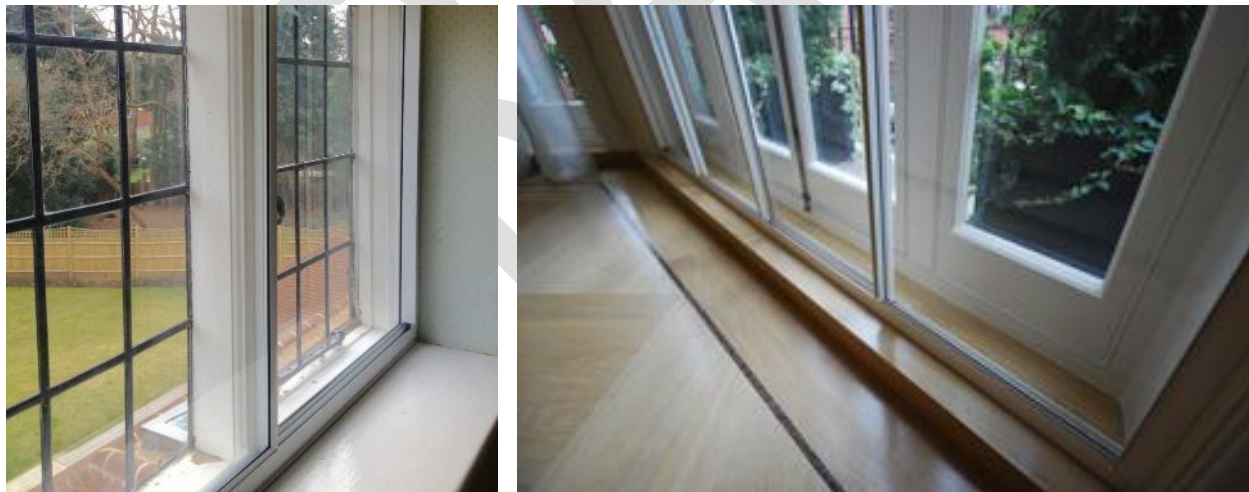
Figure 7: Secure secondary windows glazing.
