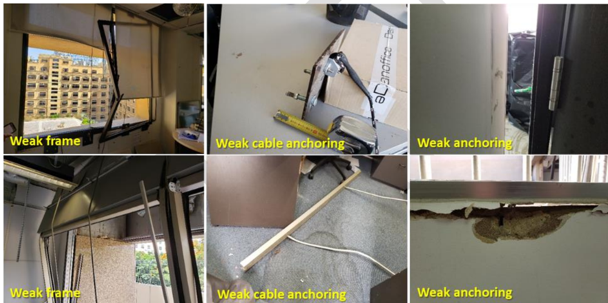
Figure 24: Damages in windows after the blast in Beirut.
