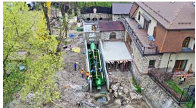
Figure 2. A challenge during the installation of the Archimedes' screw was its transportation from the semi-trailer to the channel because of high trees located in the immediate neighbourhood
