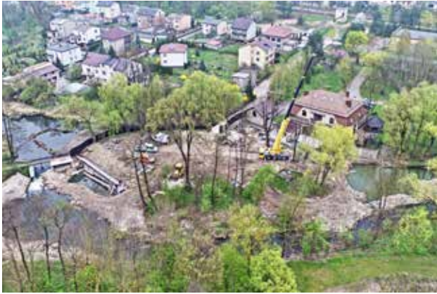
Figure 4. Construction area during the installation of the Archimedes' screw. The old hydro-technological system supplemented with the newly built fish pass is visible
