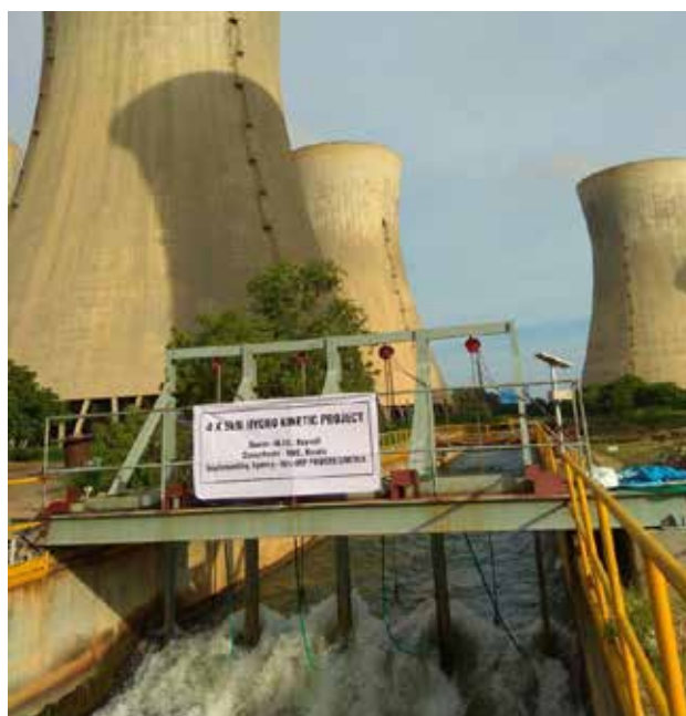
Figure 7. Neyveli Lignite Corporation kinetic hydropower plant at Neyveli, India
