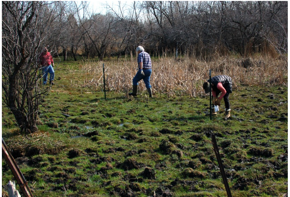
Above: UNPS members and volunteers Larry England (left), Ty Harrison (center), and Amy Defreese (right) installing barbed wire for an enclosure to protect a population of the Threatened Ute ladies'-tresses orchid in Salt Lake County. The Russian olive at left was later cut down by Blake Wellard using a hack saw. Below: the seasonally flooded wetland site being fenced. Photos by Tony Frates.
