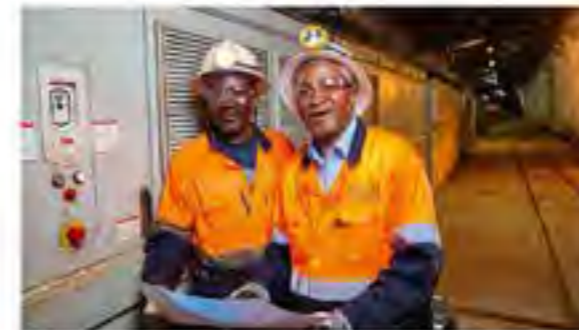
Prince Kaomba, Electrician (left), and Paul Dikwenda, Mining Manager (right), looking at diagrams of the 17.5-megawatt variable speed drives for the five high-volume water pumps installed on Kipushi’s 1,200-metre level.
