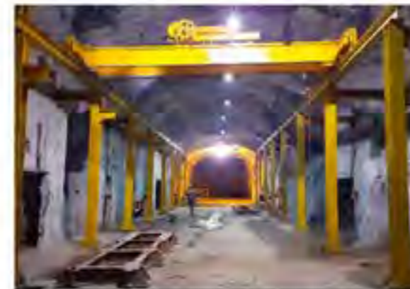
Kipushi’s newly installed 40-tonne capacity overhead crane at the 850-metre level.
