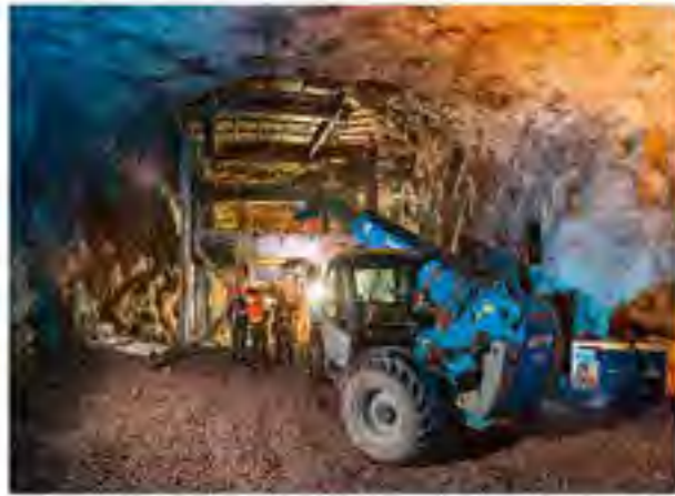
Construction is nearing completion on the underground ore transfer station, part of the ore-handling infrastructure at the Kakula Mine.
