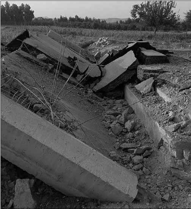
Figure 19. ADB provided $30 million for reconstruction of Kabul-Kandahar Highway that now lies in ruin
