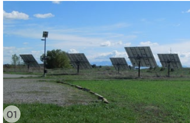
01 Photovoltaic panels at Wetland Discovery Point
