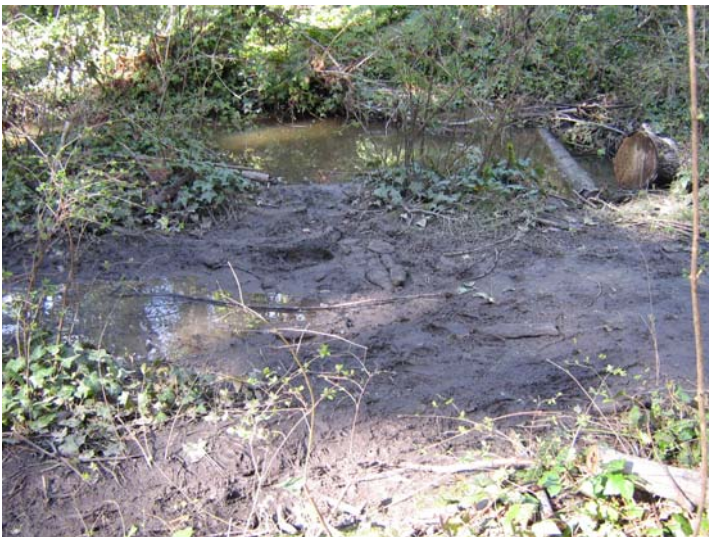
Figure 21. Erosion of Stream Bank Adjacent to Trail
