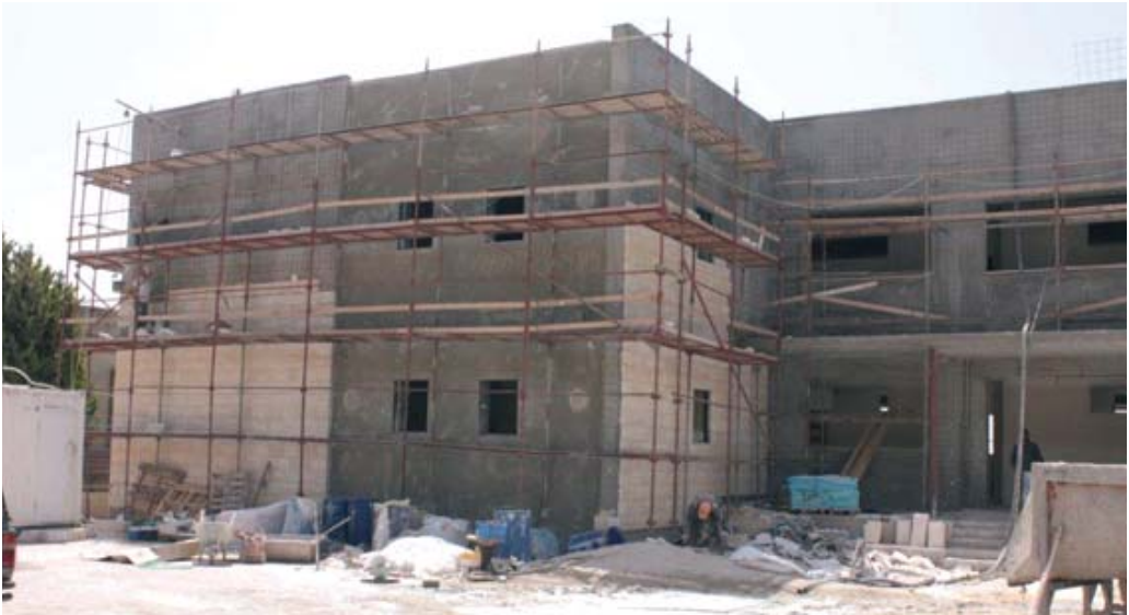
Building site in Rameh (Galilee) of the Latin Patriarchate high school. BELOW: entry to the monastery of the Sisters of the Rosary of Aboud (Palestinian territories) next to the parish church.
