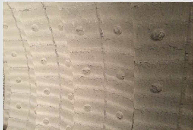
Fig. 2.1-2 ‘Coated’ mill internals
