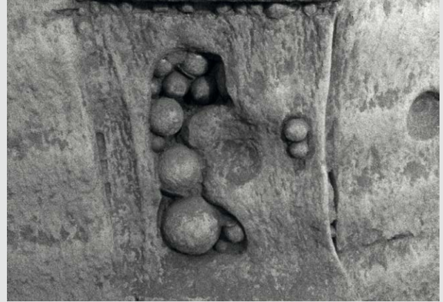
Fig. 2.1.3-1 Damage to the lining
