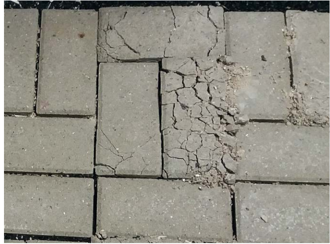
Fig. 3.4.16-2 Fragmentary scaling as a result of face concrete damage at the edges of individual concrete paving blocks
