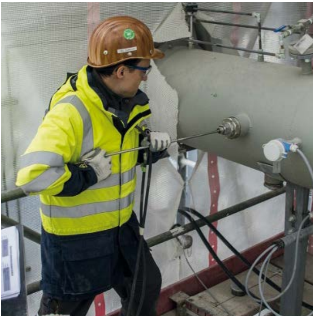
Fig. 3.2.4-3 VDZ measurements taken during trials of the oxyfuel clinker cooler prototype in a cement plant as part of the CEMCAP research project 3)
