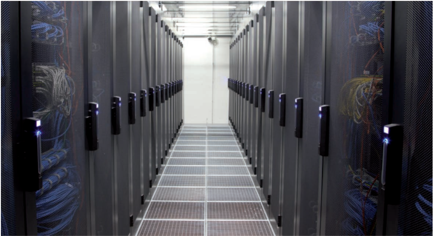
@Lock™ solution with MLR handles in a co-location datacenter
