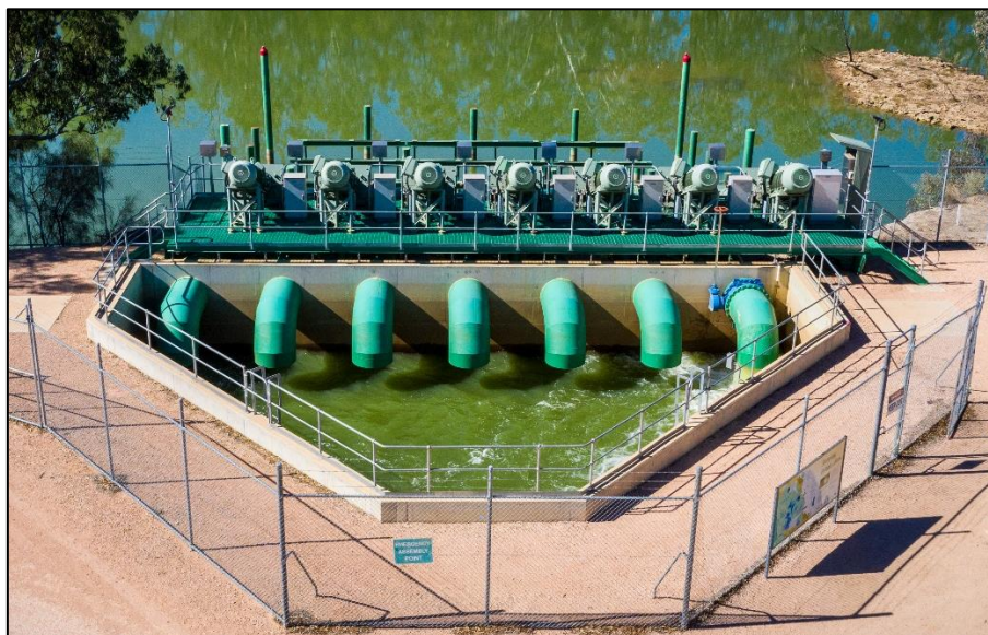
Messengers pump station (Source: MCMA)
