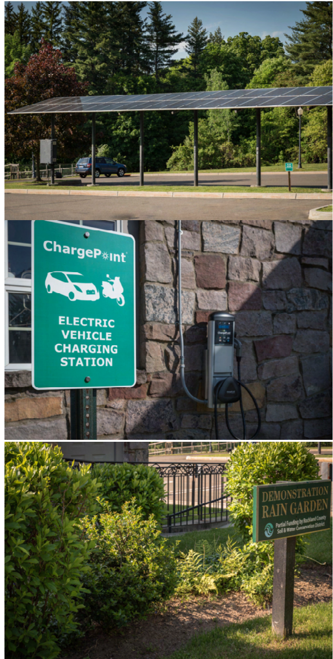
Photovoltaic system, electric vehicle charging station and demonstration rain garden at Village Hall.
